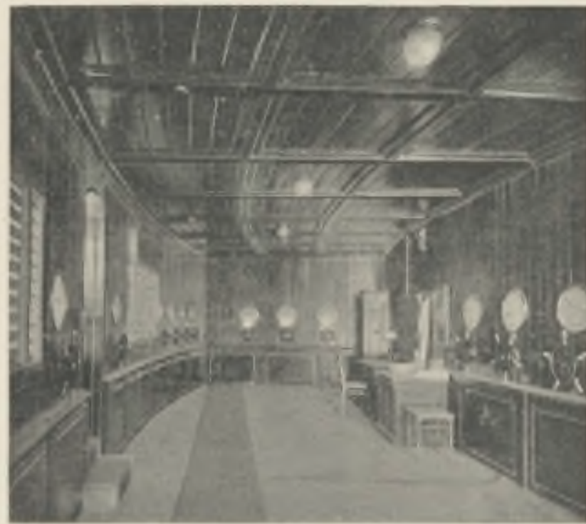
COURT THEATRE, VIENNA. FIG. 616. VIEW OF HEATING AND VENTILATION CONTROL ROOM.
