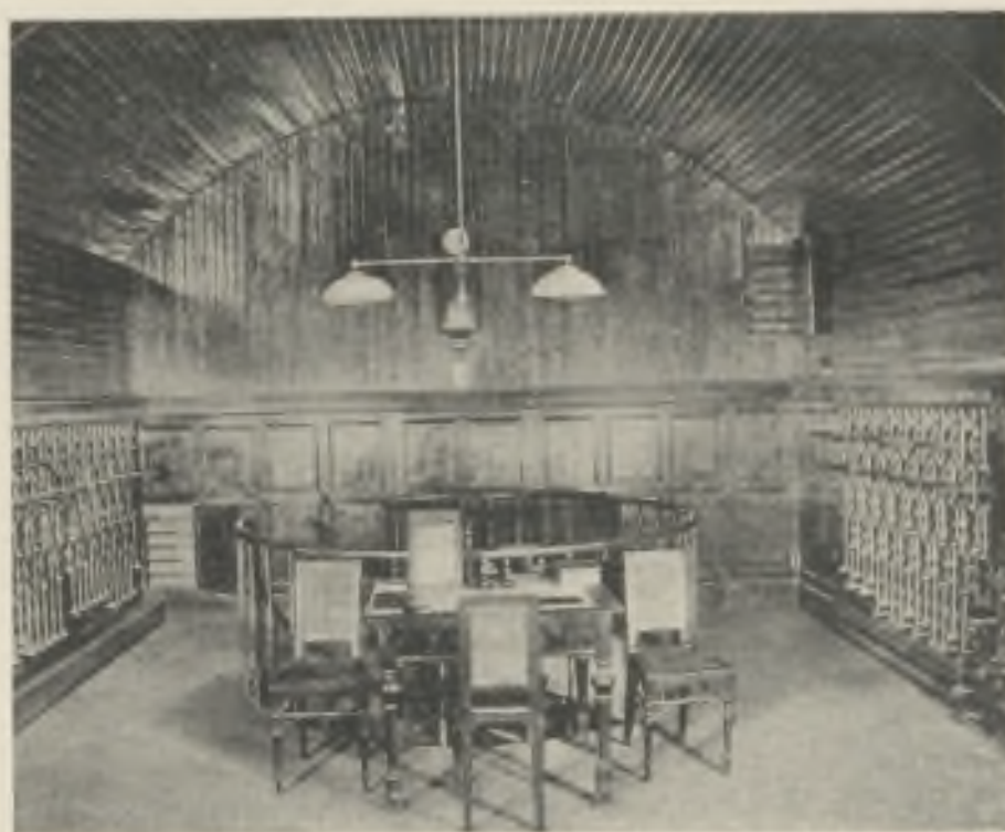
COURT THEATRE, VIENNA. FIG. 60. VIEW OF MAIN SWITCH ROOM.
